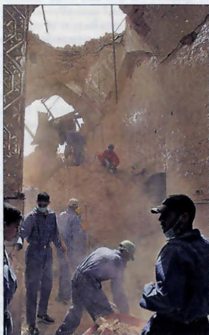
Rebuilding in a war zone is expensive.
